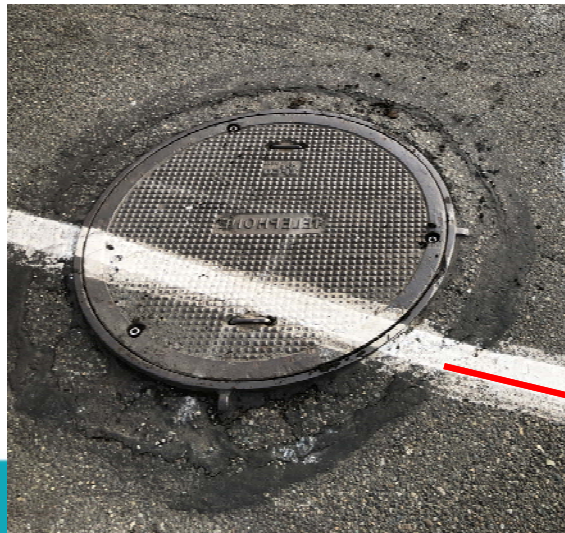
Settlement Around Utility Lid
